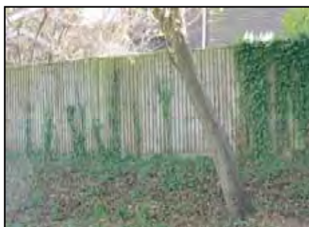
A close boarded panel fence
